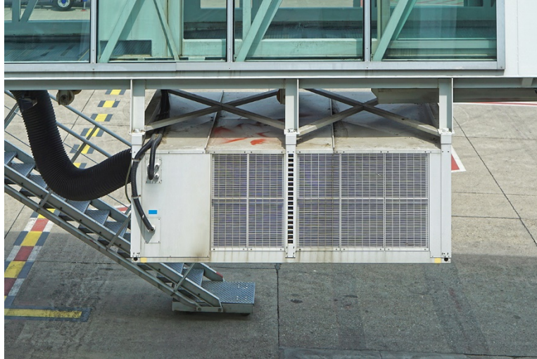
Figure 4.5 A Pre-Conditioned Air (PCA) System Attached to a Jet Bridge
